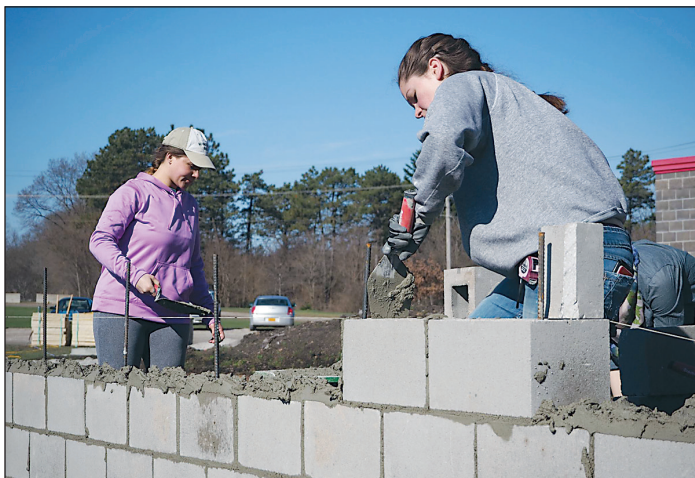
Kaela Burmeister of Humboldt (right), an architecture student at Iowa State University, is shown laying block as part of the renovation of the Cap Timm baseball field at ISU.
